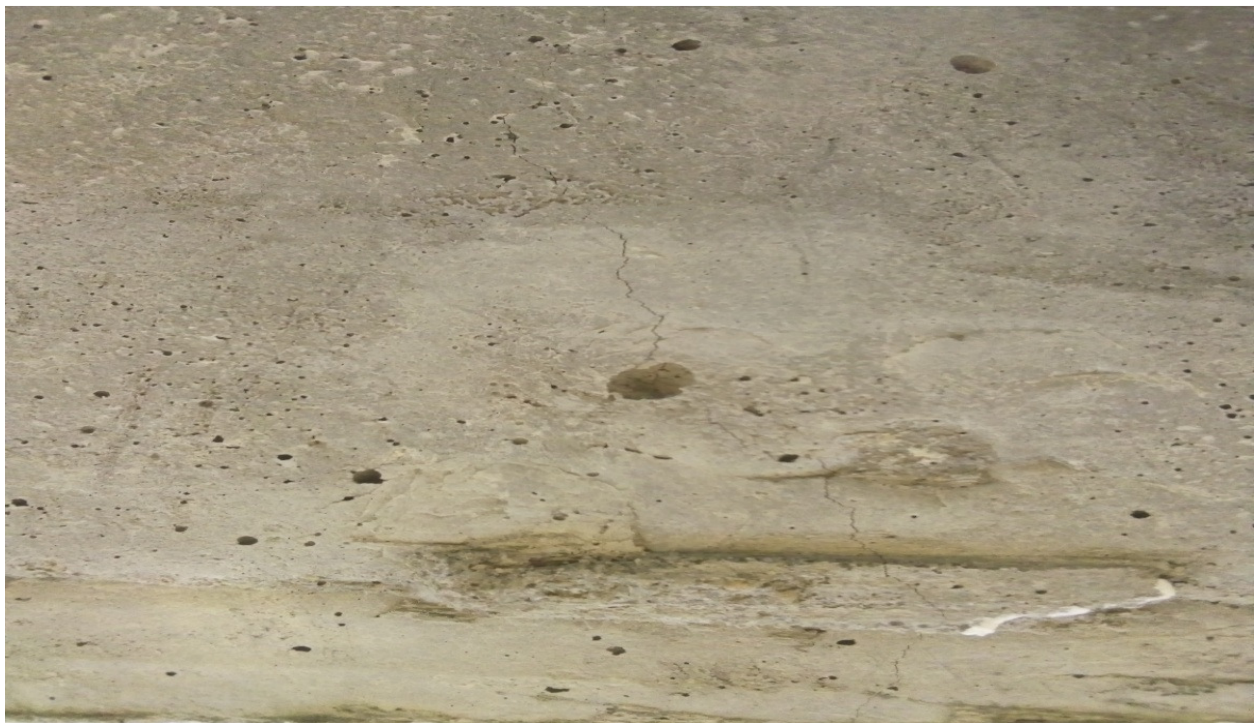
Figure 5: shows a crack appeared on D350-10%
