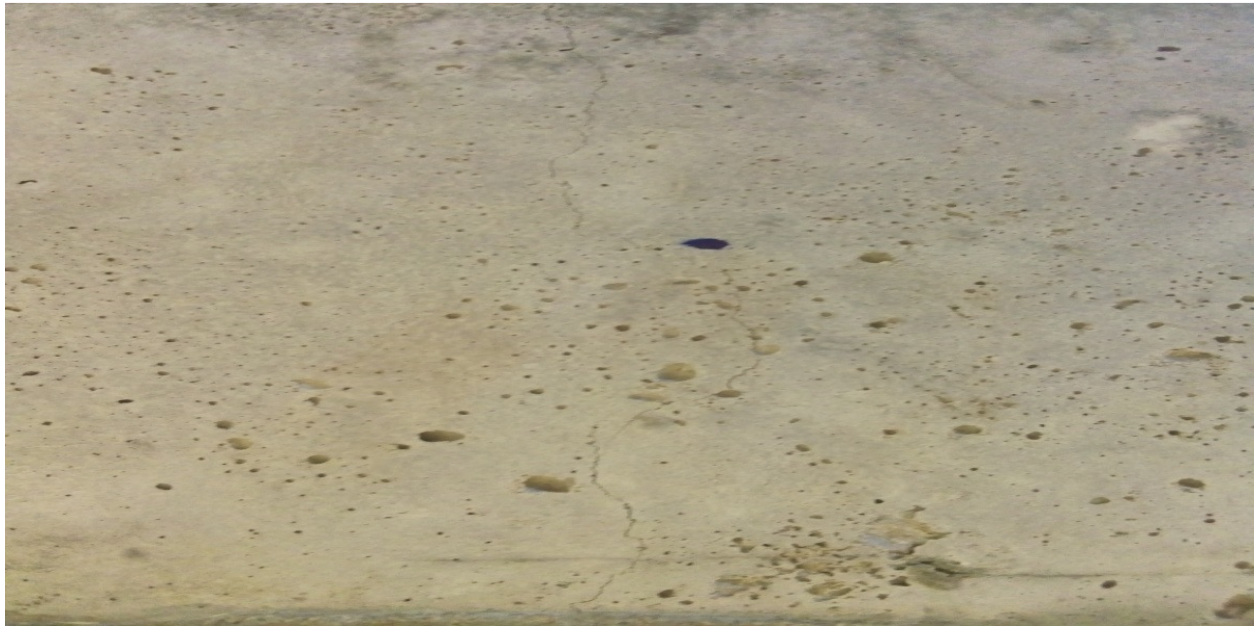
Figure 4: shows a crack appeared on D350-0%
