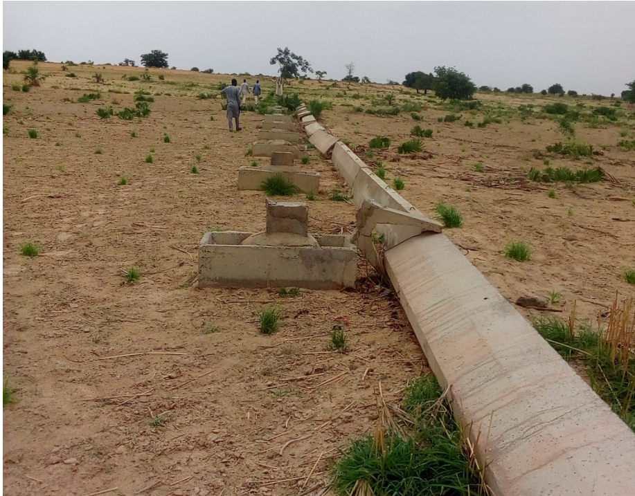
Figure 5: One of the collapsed tertiary irrigation canals at the Sabke dam irrigation sites
